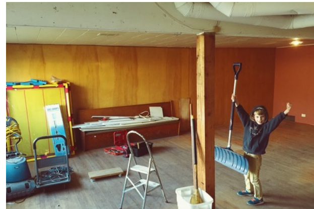
Maximus in the section of the basement that will be the new children's classroom.
